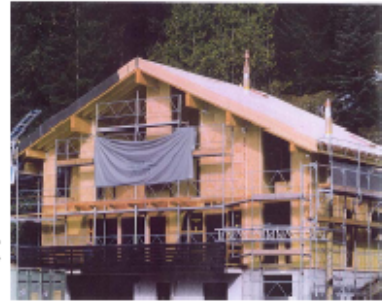
(top right) A building under construction showing 3 storey load bearing Steko walls.
